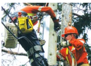
A crew from Waterloo North Hydro on the job in Elmira as part of a back lot pole replacement project
